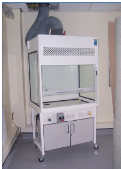
■ Fume cupboards, the most important pieces of equipment, must be ducted.
